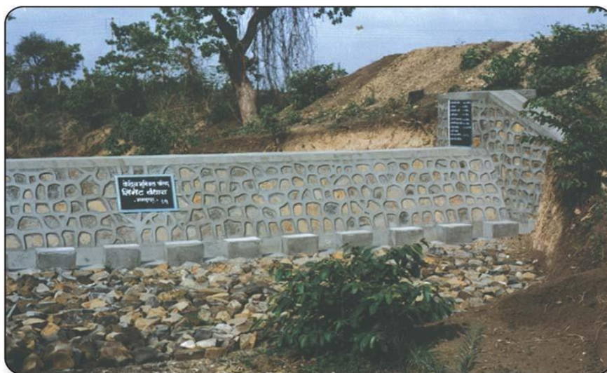
Figure 17: Field photo of a Check dam
