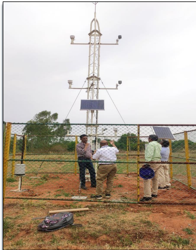
AMS Tower Installed in the Field
