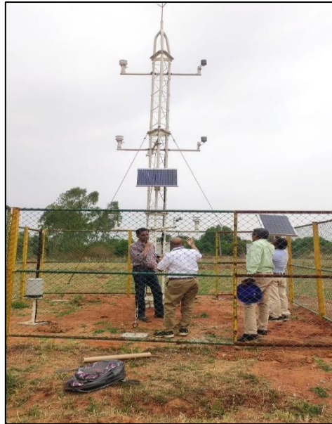
AMS Tower Installed in the Field
